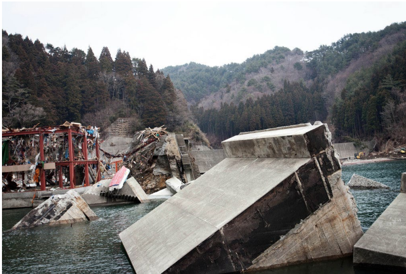
Figure 48: The Kamaishi breakwater, which failed during the 2011 Japanese tsunami (NY Times)
