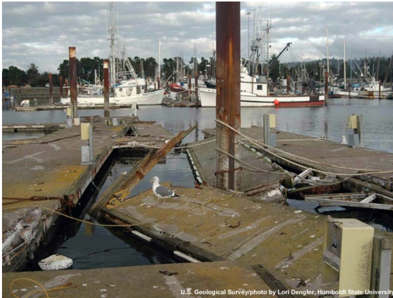
Figure 46: Broken docks in Crescent City, CA from the 2006 Kuril earthquake ( USGS 2006 ).
